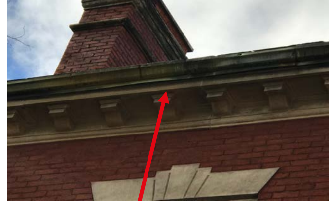
Exterior work needed
