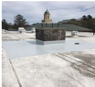
Roof Upgrades needed
