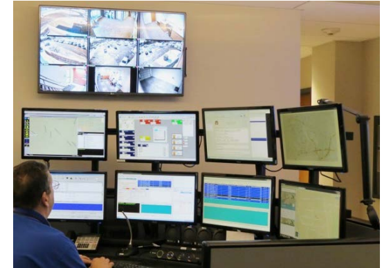
Dispatch Control Equipment
