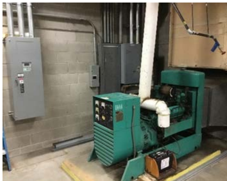
Outdated Emergency Generator
