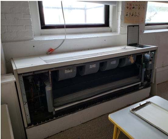
Picture 1 - Typical Classroom Unit Ventilator
