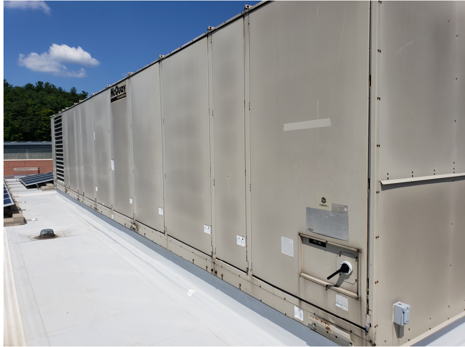
Picture 3 – Roof Top Air Handling Unit
