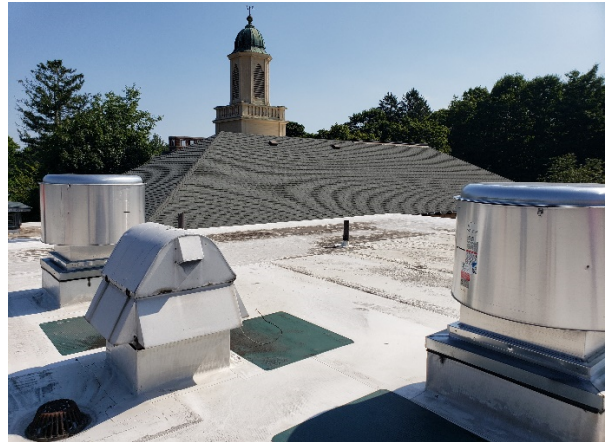
Picture 2 – Roof Top Exhaust Fans
